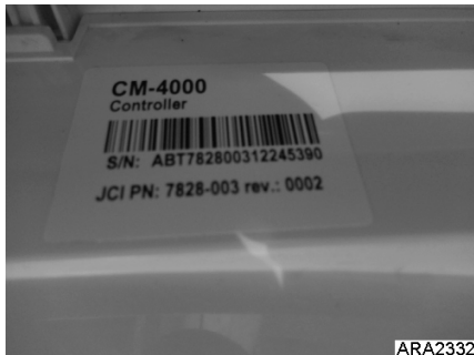
Label on Controller
