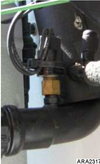
Low Pressure Cutout Switch Installed
