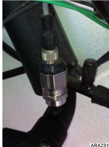
Suction Transducer Installed
