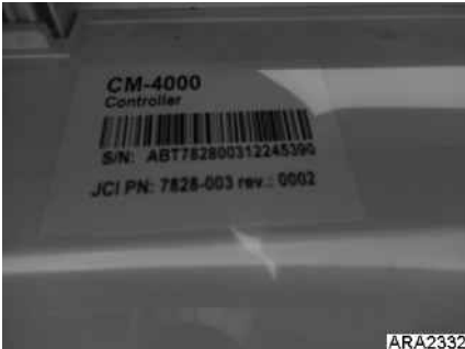
Label on Controller
