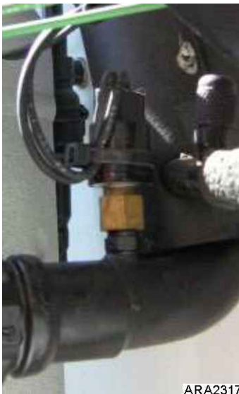
Low Pressure Cutout Switch Installed
