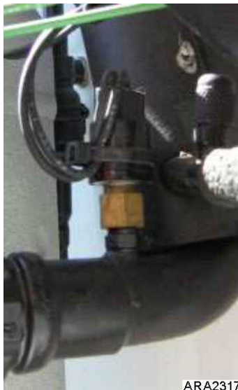
Low Pressure Cutout Switch Installed
