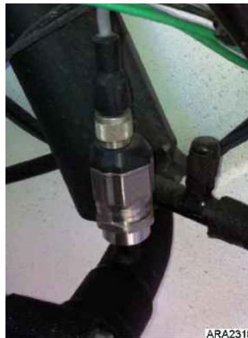
Suction Transducer Installed
